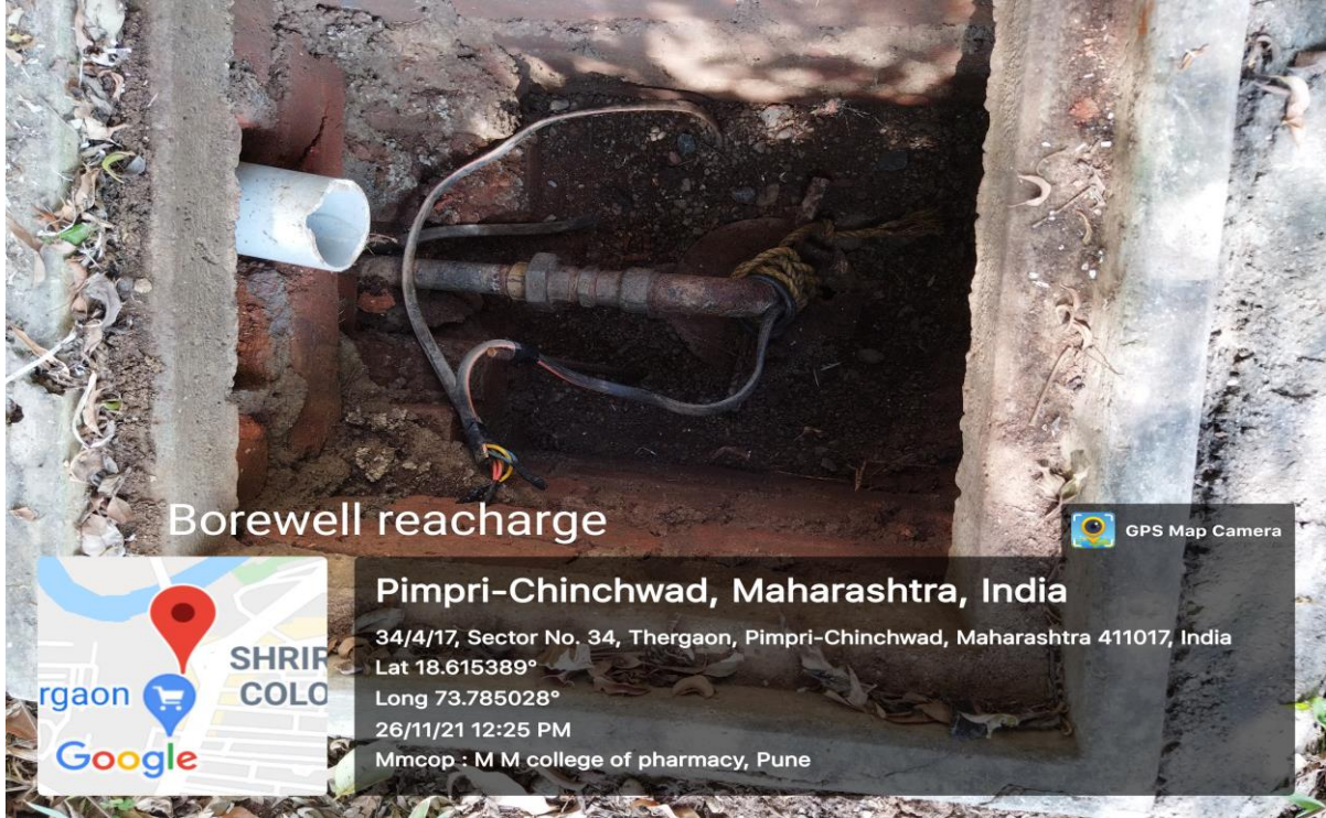
Rain Water pipe laid near the Bore well Pump for recharge
